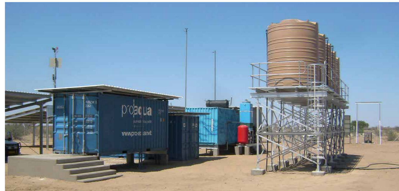
Fig. 57: Solar desalination plants in the village of Amarika. → Photo: CuveWaters project
