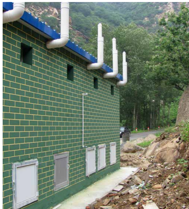
Fig. 19: New compost toilet in Huangyukou – rear view with drying chambers after construction. → Photo: Beijing Water Authority
