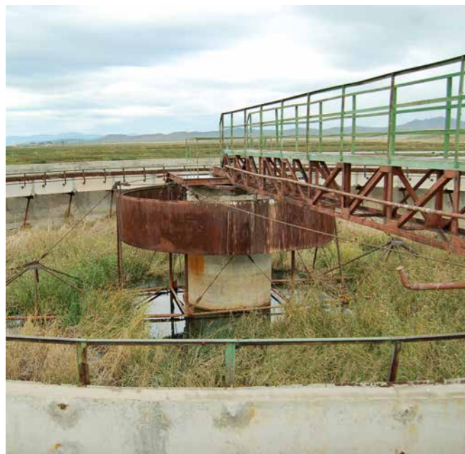
Fig. 10: Dilapidated infrastructures are often the result of inadequate governance. → Photo: L. Horlemann
