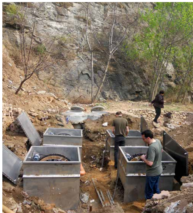
Fig. 18: Installation of the rotating biological contactor (RBC) sewage treatment plant in Taoyuan. → Photo: Beijing Water Authority
