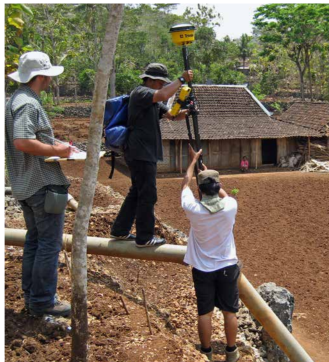
Fig. 26: Data collection as basis for simulation studies regarding the optimization of the water distribution network and its structural implementation. → Photo: KIT/IWRM Indonesia
