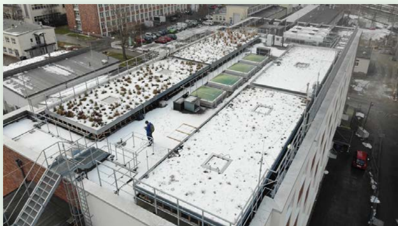
Figure: Research green roof under a snow blanket on January 18, 2021 Author: Jan Knappe
