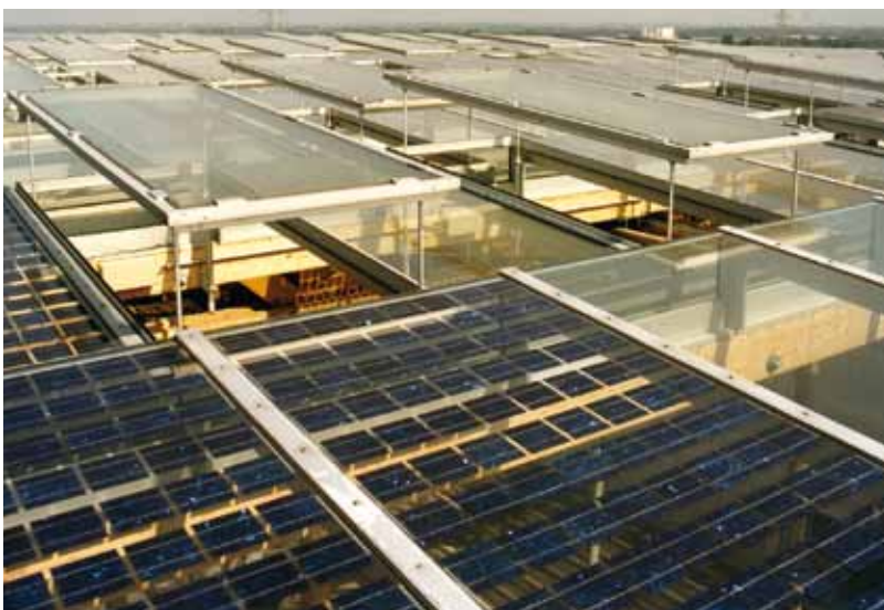
View onto the Roof of the Main Building of Revitalized Mining Facility
