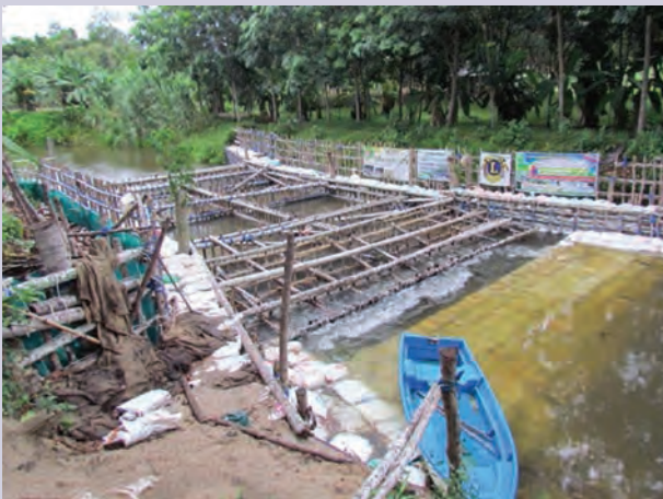
Check dams are relatively small, temporary structures constructed across a swale or channel. They are used to slow the velocity of concentrated water flows, a practice that helps reduce erosion.
